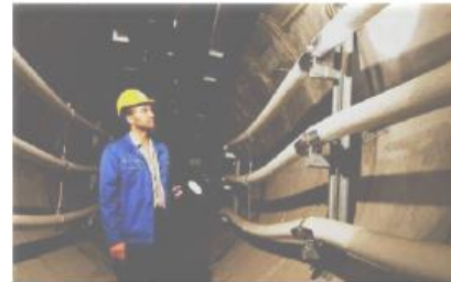
400 kV XLPE cable system
