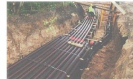
Multiple 110 kV XLPE cable systems
