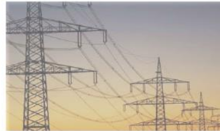
400 kV overhead line
